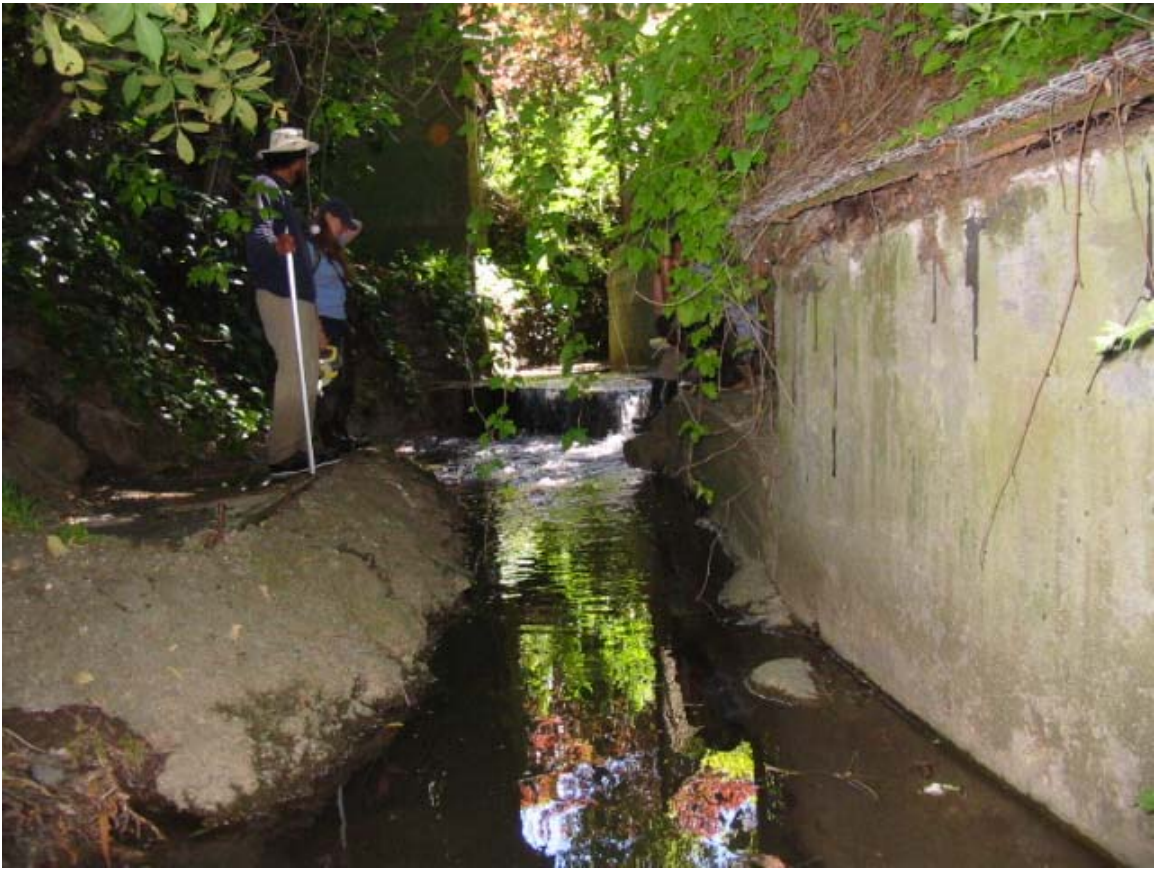
Figure 22. Concrete step, 1.6' in height, at the downstream edge a straightened concrete lined channel. The concrete channel begins at the outfall of the Monterey Avenue culvert and extends downstream for 232'.
